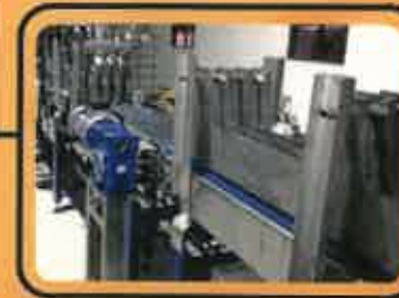
Conveyor lane diverter
